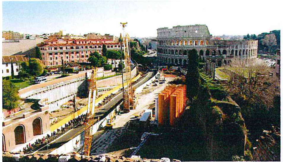
Fig. 1 - A view of the construction site of Fori Imperiali Station (central stretch).
