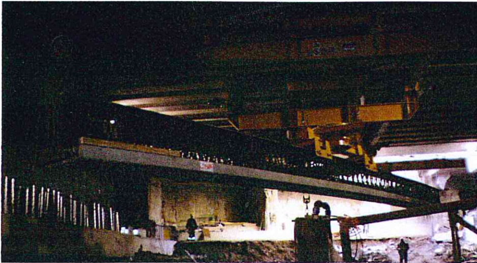
Fig. 8 – The launching carrier used to move prefabricated structures and the perimeter concrete edging.
